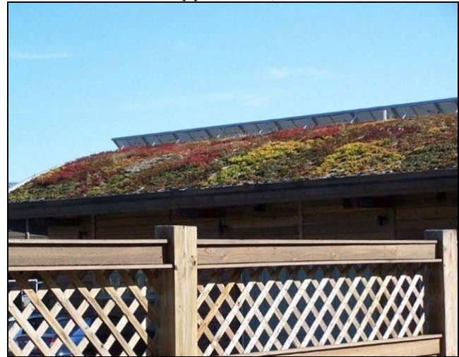
Figure 5. 45 Green roof installed on a sloped roof, Tupper Lake, NY
